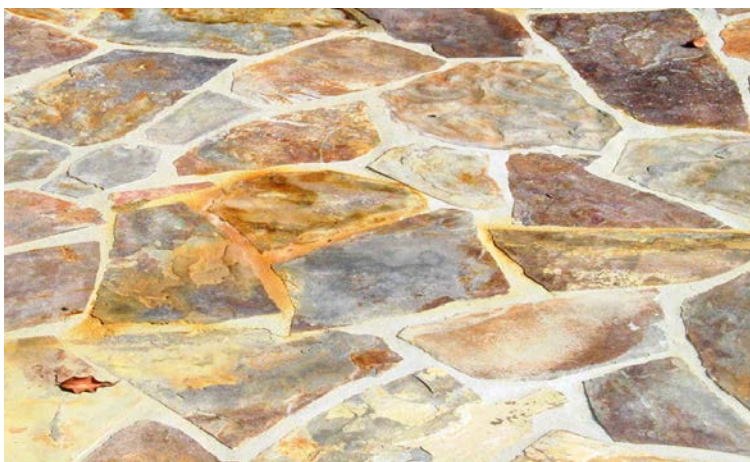
Figure 2: A closer look at the rusting of the same slate around the pool.
