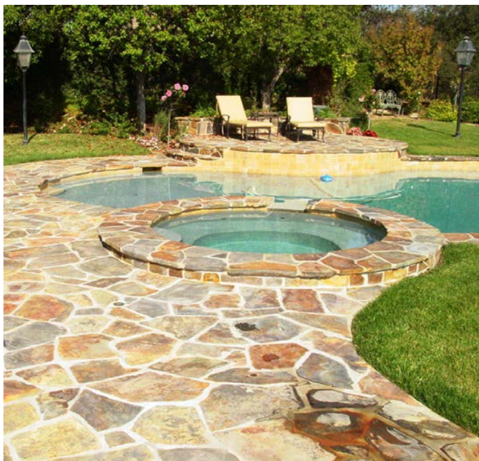
Figure 1: The above slate is high in iron content and is beginning to “bleed” a rusty stain. Some of the most dramatic colors are already ferric – they don’t react well to surface treatments.
